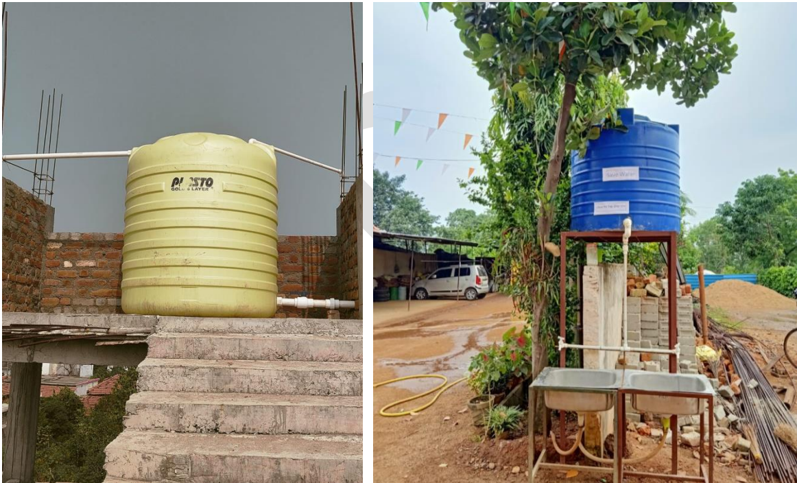
Water storing Tank and drinking water facility
